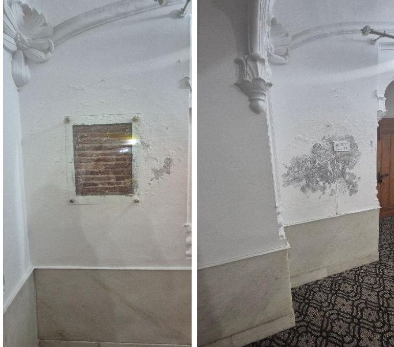
Figure 26: a) Untouched part of the Original structure; b) Irreversible actions taken on site
