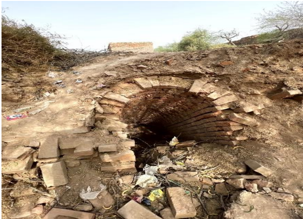
Figure 15: Underground room has been blocked due to rain
