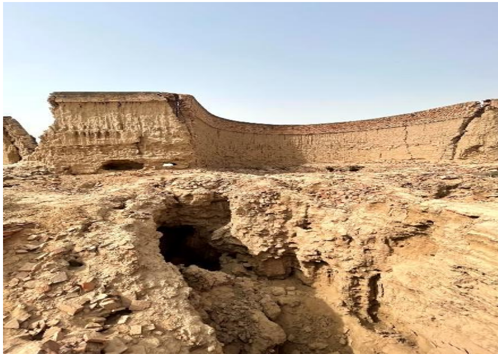
Figure 13: Rainwater penetrates surface level and percolates downward into buried structures, leading to the outer walls/bastions.
