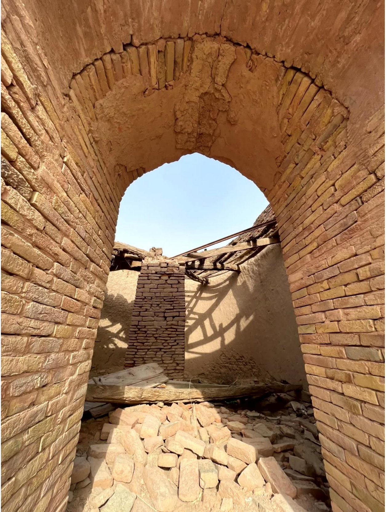
Barracks are also not in good shape.
