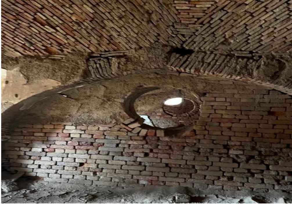
Figure 14: The roof and walls of the room have been damaged.
