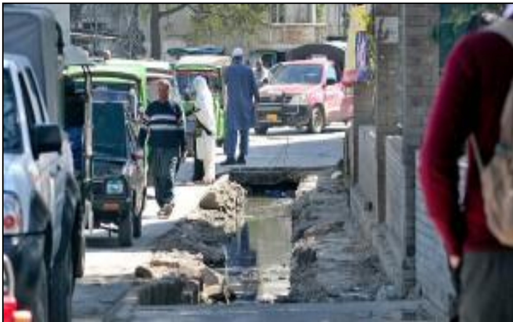
Figure 2-6: Open drain in footpath
