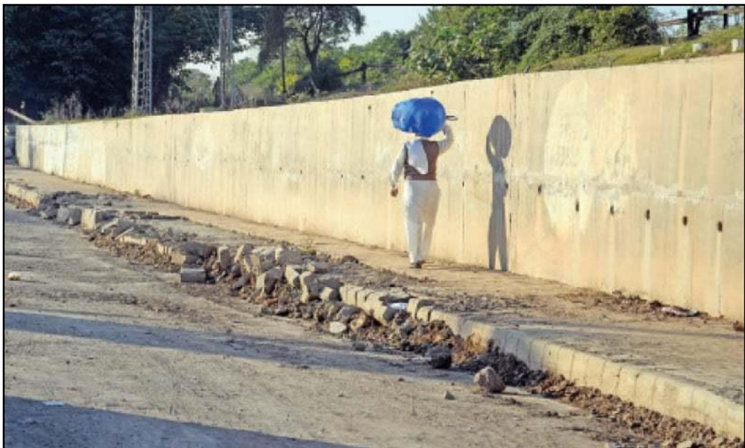
Figure 2-5: Uneven surface on footpath
