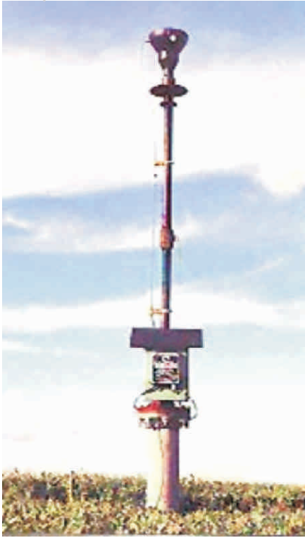
Figure 8.16: Typical candlestick type waste gas burner used to flare landfill gas from a well vent or several interconnected well vents
