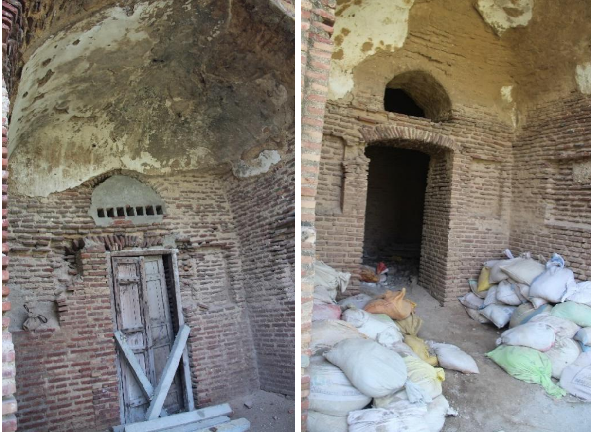
Figure 13: One of the Deteriorated Areas in Sarai
