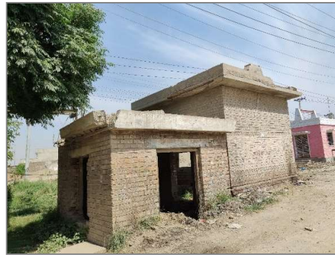
Abandoned tube-well on the Qutab Canal. The structure is severely deteriorated and classified as Failed condition.
