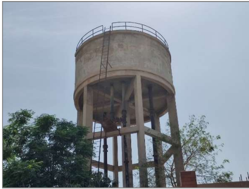
Abandoned OHR of 30,000 Gallons capacity. The poor structural health is clearly evident from the picture above.
