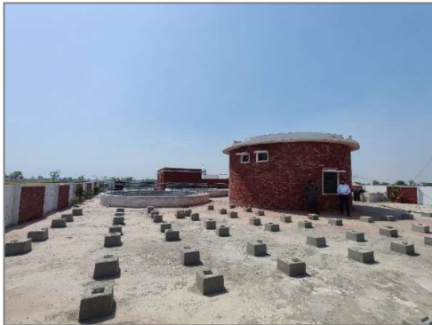
Under Construction DS Fatehpur Road. Solar system is proposed to be installed at the two Under Construction Disposals.
