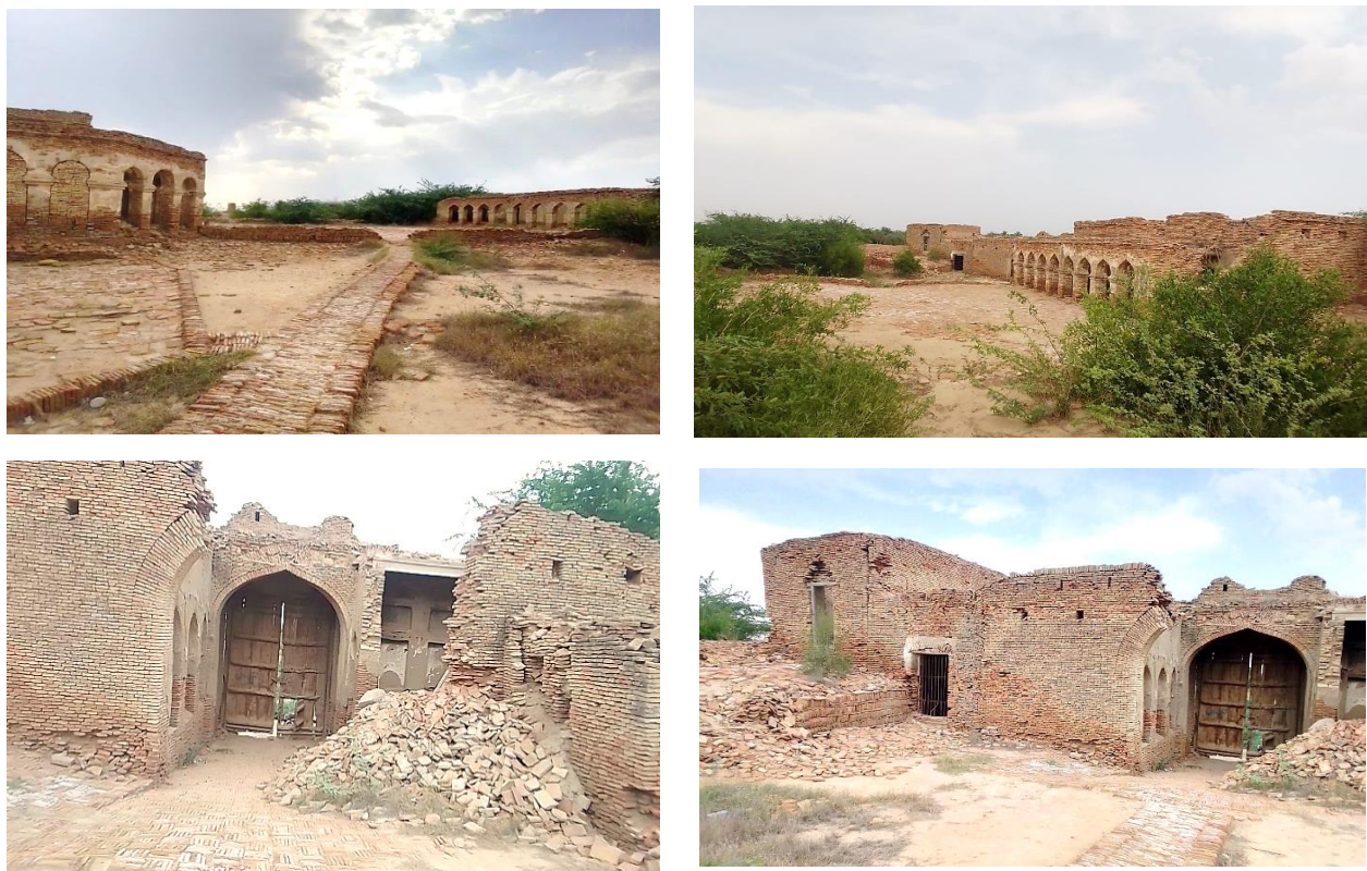
Figure 47: Dilapidated condition of Harrand Fort
