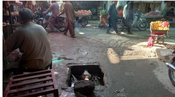
Figure 80. Open Manhole in Main Bazar
