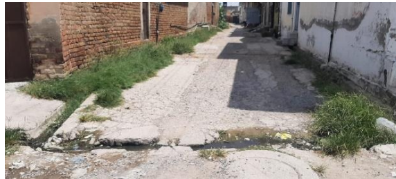
Figure 60. Unpaved and broken streets in Mohallah Bhattian
