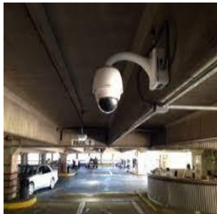
Figure 94. CCTV Cameras for Security and Monitoring
