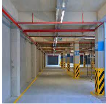
Figure 95. Fire alarms should be set in the plaza.
