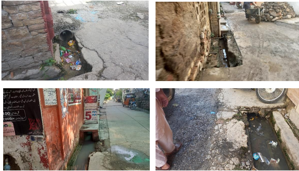
Figure 79. Open drains in residential areas
