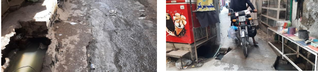
Figure 56. Open Drains and Broken Streets in Old Bazar.
