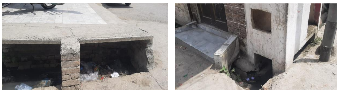
Figure 75. Open Drains in Some Residential and Commercial Areas in Attock
