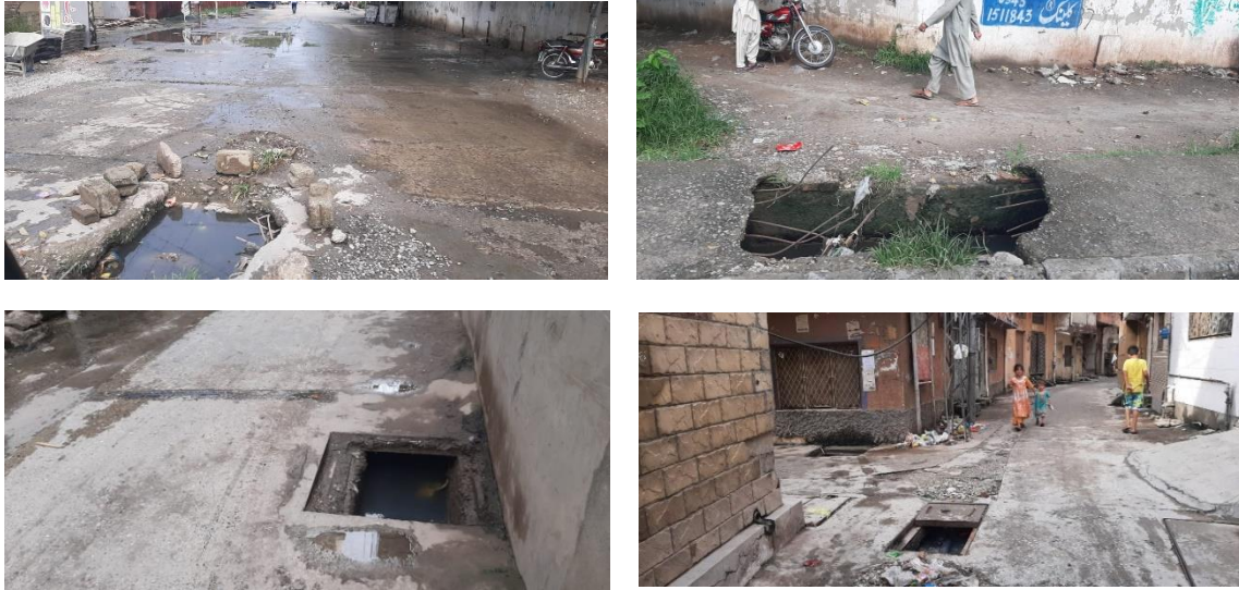
Figure 39. Open manholes in different residential areas.
