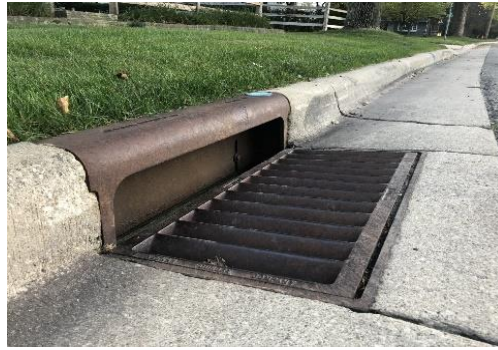
Figure 104. Cover open drains that exist at sideways of streets and roads in Raja Bazar area
