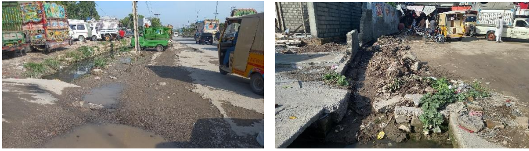
Figure 82. Rainwater remains clogged in broken patches of road
