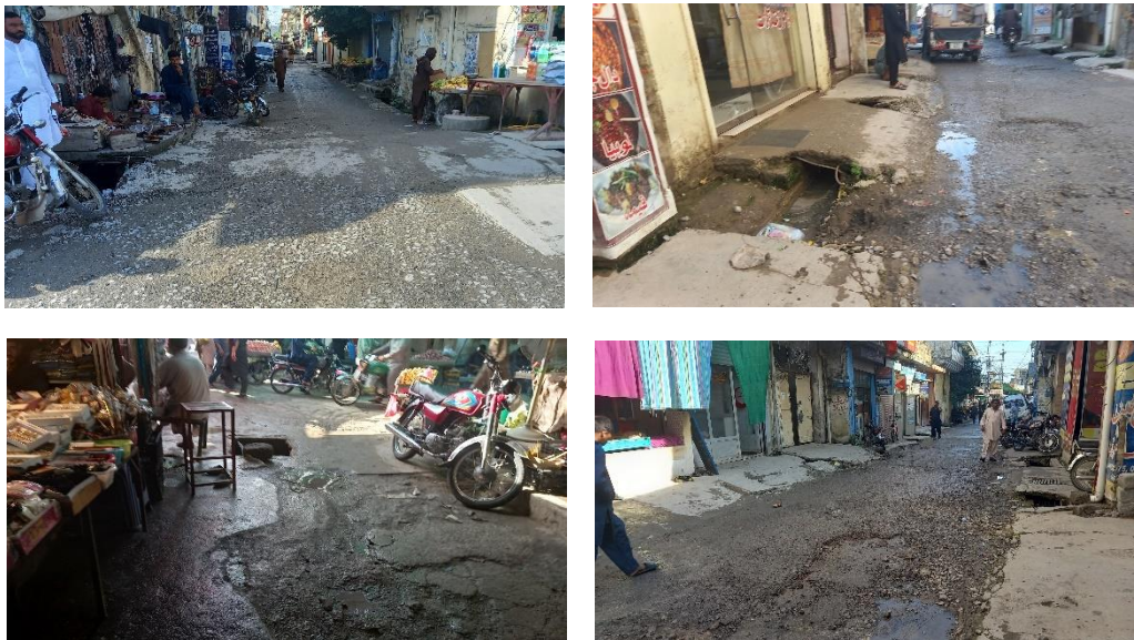
Figure 77. Broken Streets in residential and commercial areas in Hasan Abdal.
