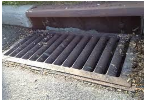
Figure 135. Cover manholes and open drains
