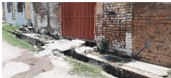
Figure 61. Open drains at sideways of a broken street
