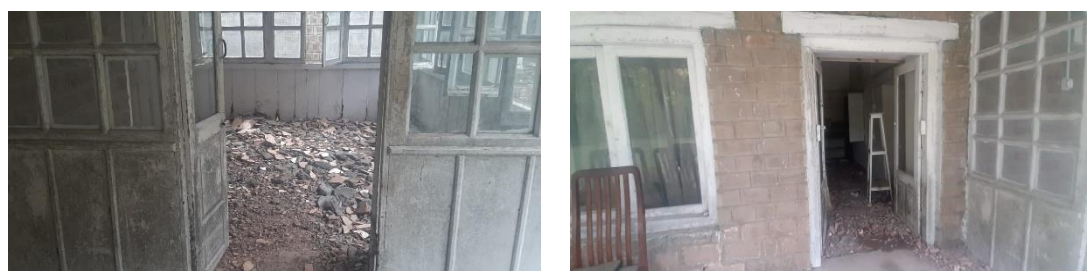
Figure 54. Poor Condition of the Rooms.
