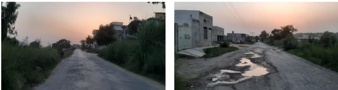
Figure 66. Broken patches of Main Road
