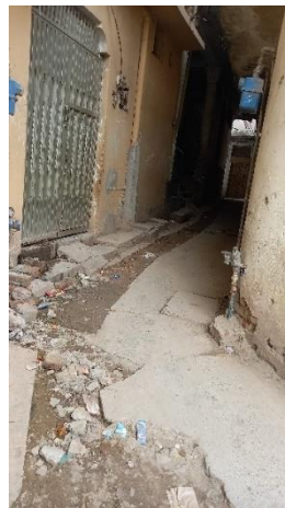
Figure 40. Condition of streets in Ghareebabad
