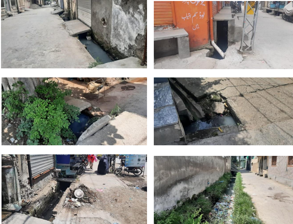
Figure 70. Open Drains in Residential and Commercial Areas
