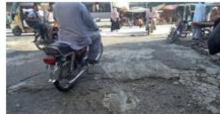
Damaged condition of roads connecting slums
