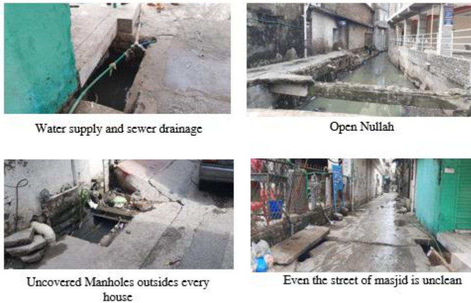
Figure 138. Existing Situation in Sadiqabad, Rawalpindi.
