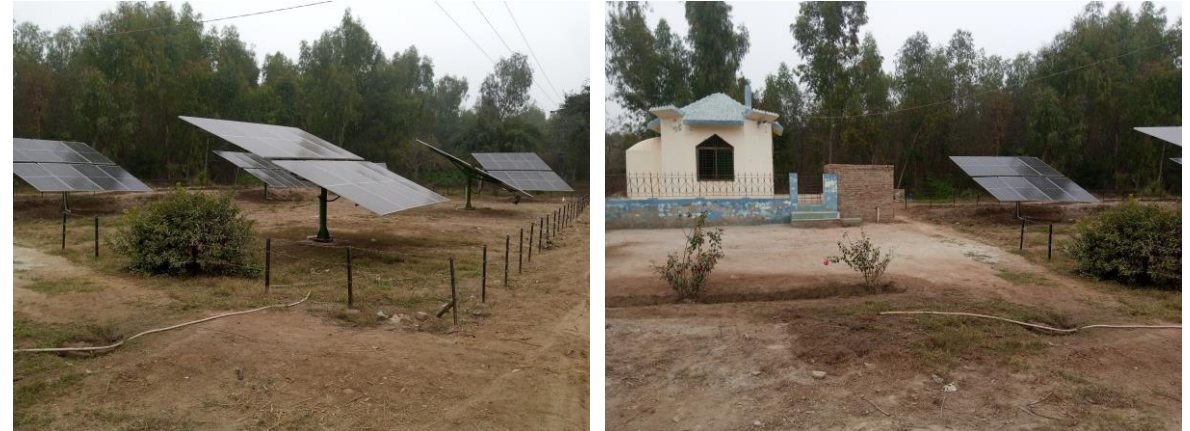
Existing Tube well in Depalpur Forest
