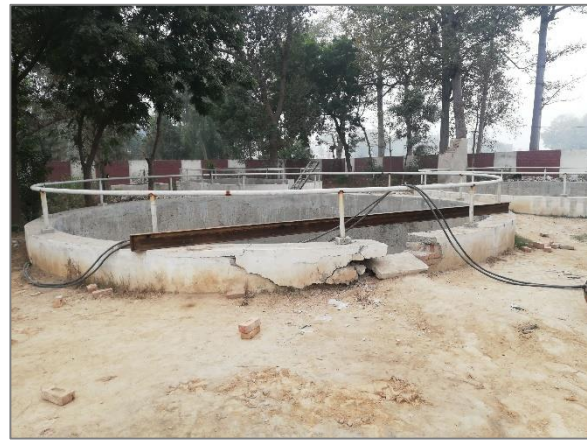
Wet Well of 2/4 L Disposal Station
