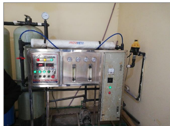
Allama Iqbal Road RO Filtration Unit Installed in 2020. Satisfactory condition of the FP was observed
