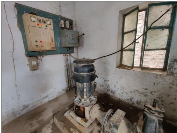
A tube well in Chak 19/SP of Pakpattan. Installed in 2000, the TW in Chak 19/SP is still functional but at the verge of its design life as evident from the picture above
