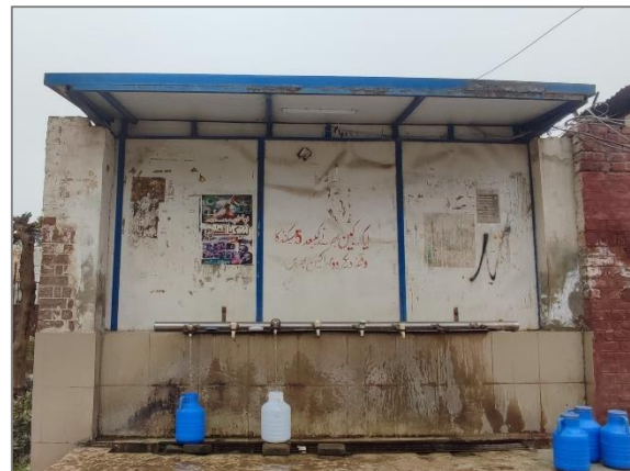
Filtration Plant located in Press Club Sahiwal needs immediate rehabilitation
