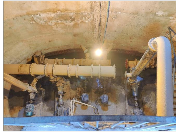
Pumping machinery at the main Disposal Works Tiba Sherkot in MC Pakpattan.
