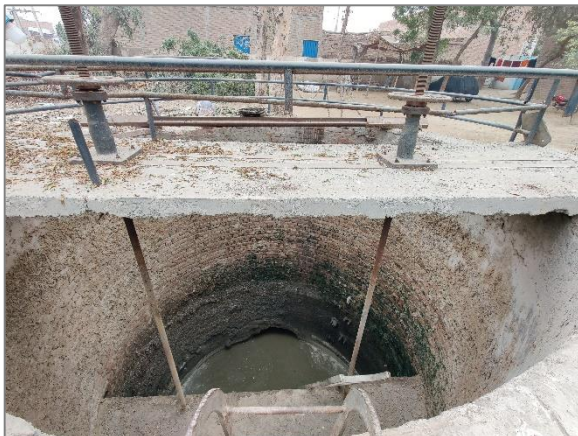
Condition of Wet Wells at Disposal Works Tiba Sherkot in MC Pakpattan.
