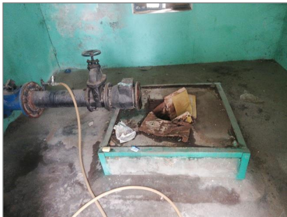
Non Functional Tubewell TW#03 due to bore failure
