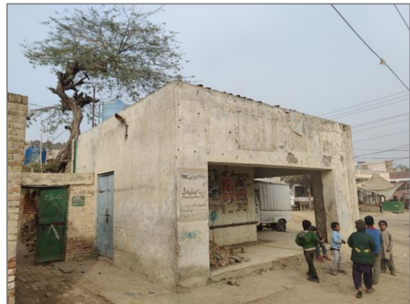
Rural Filtration Plant in Pakpattan. An abandoned Rural Water Supply Scheme and Filtration Plant in Chak 59/EB of Arifwala Tehsil
