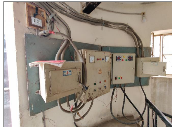
Condition of electrical panels at Disposal Works Jamal Town in MC Pakpattan.
