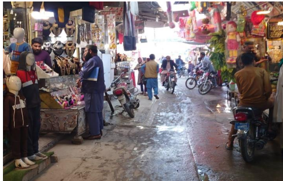
Poor Street Condition
