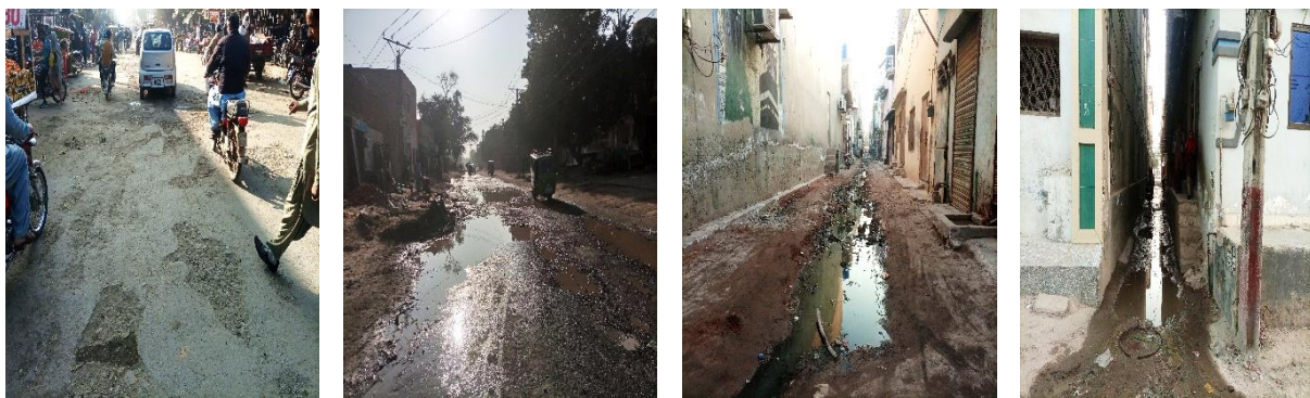
Figure 43: Condition of Streets in the residential area and in Main Roads located near High Street Road
