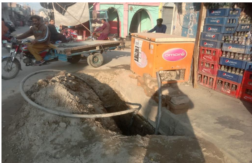
Figure 105: Poor quality broken infrastructure of water supply
