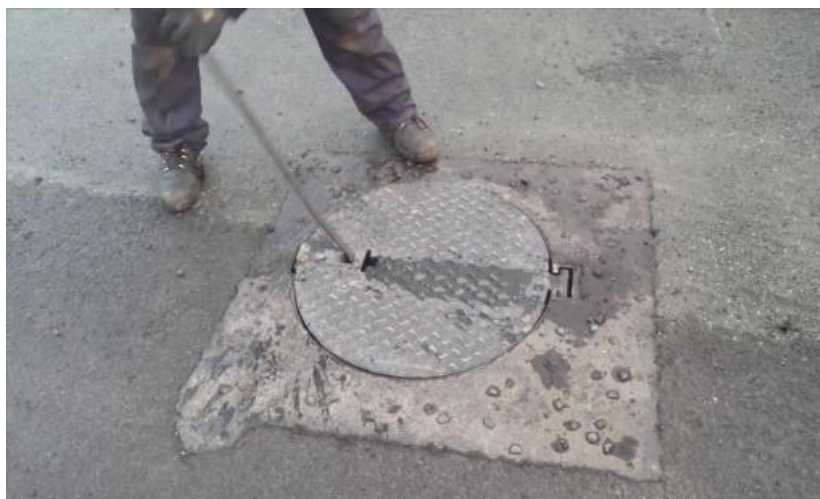
Figure 74: Cover open drains that exist at sideways of streets and roads in Bazar
