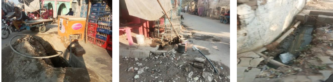
Figure 55: Poor Conditions of Water Supply Infrastructure, Pakpattan.
