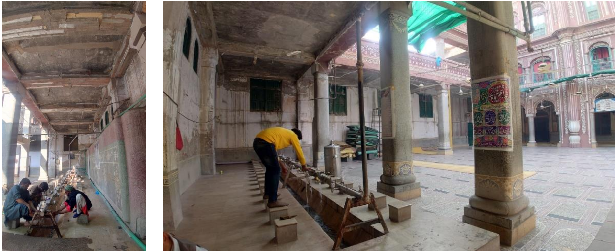
Figure 25: Vandalism on the walls inside, Poor Condition of the ablution area.
