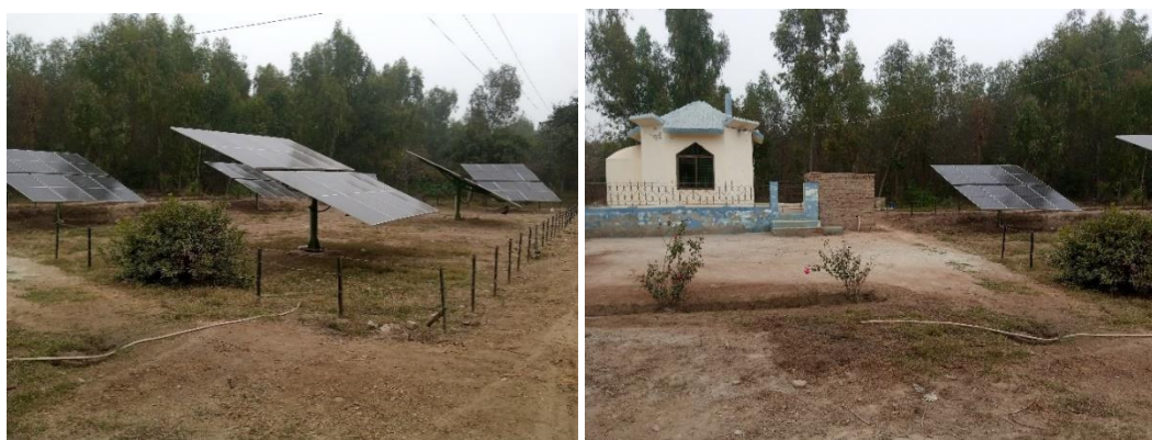
Figure 46: Existing Solar System and Tube Well in Depalpur Forest Plantation
