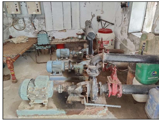
Inside a pump house, H Block Water Works
