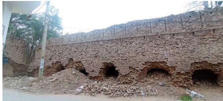
Figure 14: Arched walls of Tulamba fort in dilapidated condition
