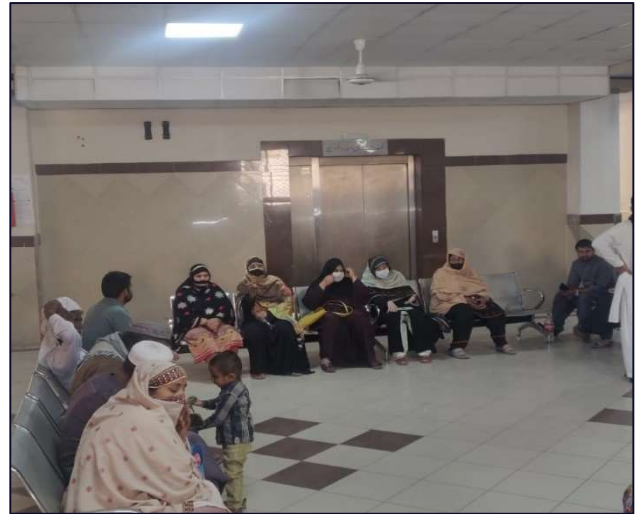
Non-functional lift to take patients to operation theater in DHQ Multan (estimated cost will be 9-10 million)
