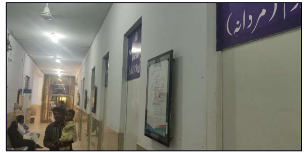
Toilets located in the middle of patient waiting areas, can be replaced by OPD rooms
