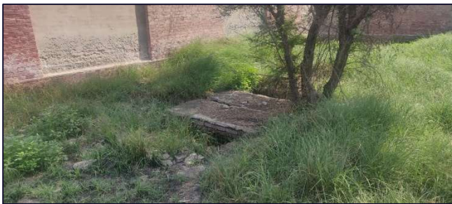
Repetitive drainage problem, caused damaged to boundary wall in BHU Chak 355 W/B
