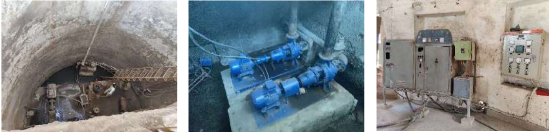
Figure 57 Condition of Electro-Mechanical Components of Sewerage Infrastructure
