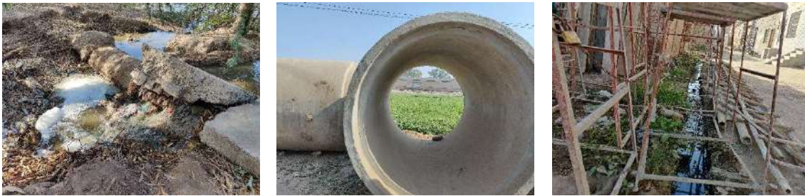
Figure 58 Condition of Sewer Lines and Distribution Infrastructure
