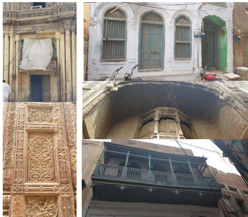
Figure 91: Dilapidated condition of Heritage Buildings
