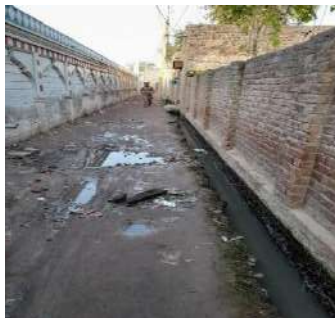
Open Sewerage Lines
