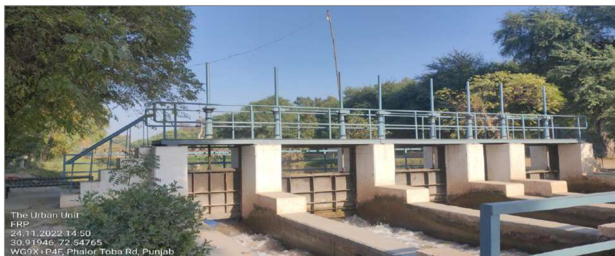
Figure 15: Mechanical gates for controlling water at a canal in Bhagat Sub-Division, T. T. S.
