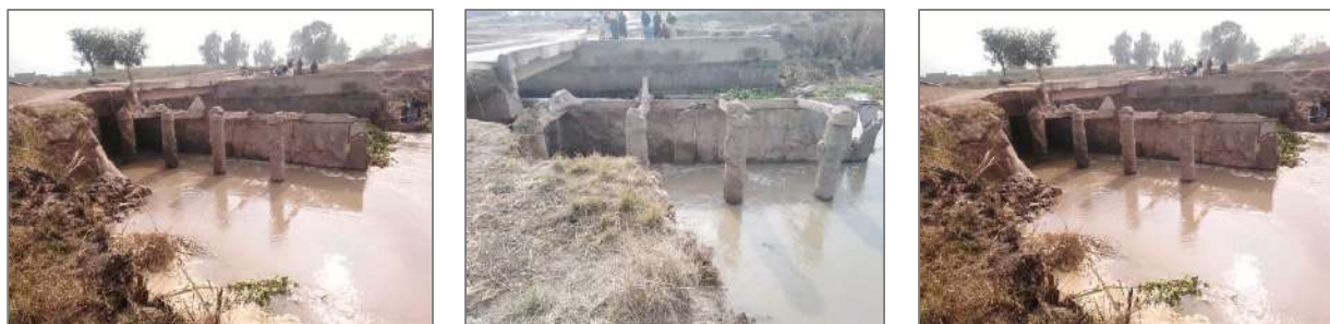
Figure 5: Condition of Canal Fall in Chiniot District
