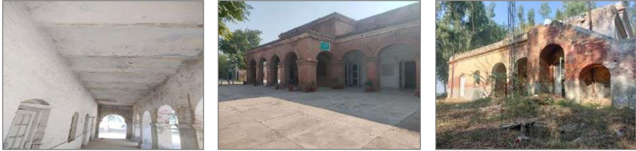
Figure 6: Condition of rest house and office of irrigation department
