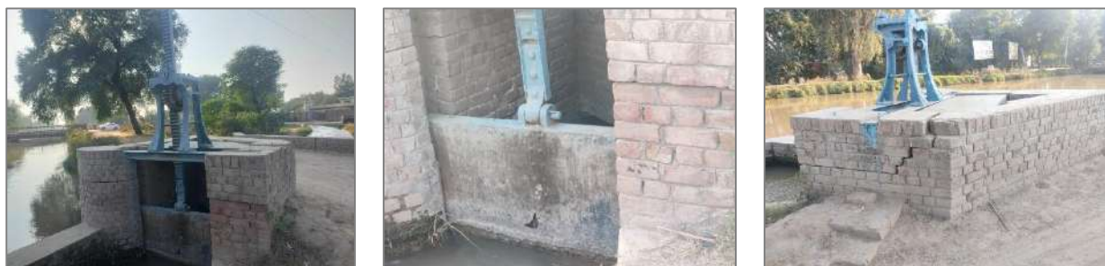
Figure 4: Condition of gates of cross and head regulators
