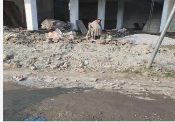
Poor drainage and footpaths
