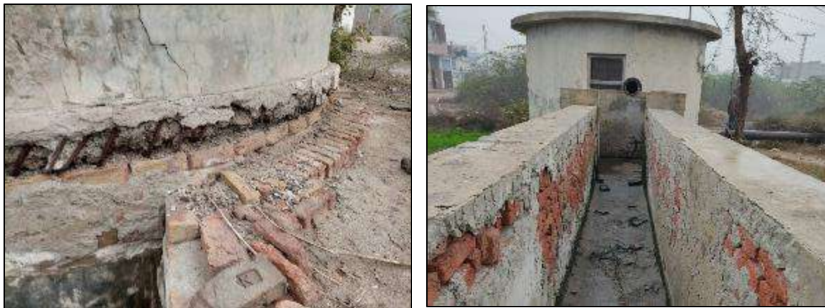
Figure 36: Condition of Sludge Carrier of Disposal Station Khushab
