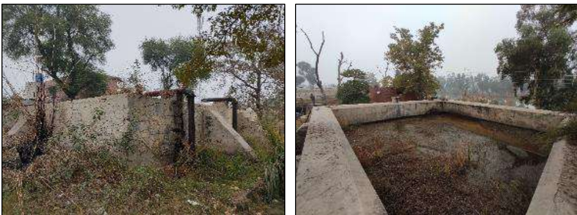
Figure 26: Slow Sand Filter at Water Works Khushab in deteriorating condition
