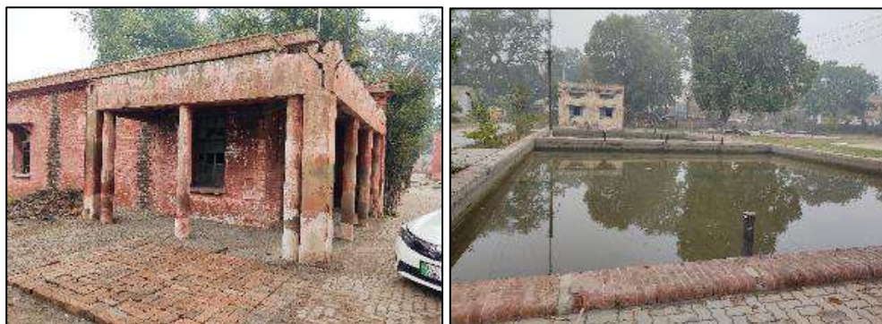
Figure 13: Damaged civil structure and Sand Filter bed at Main Water Works Sargodha
