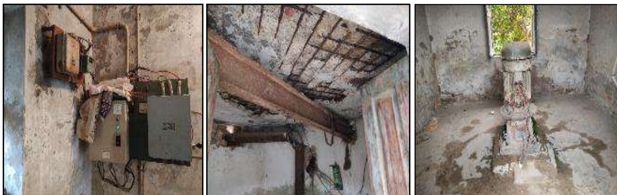
Figure 5: Example of Condition of WSS Infrastructure- very Poor
