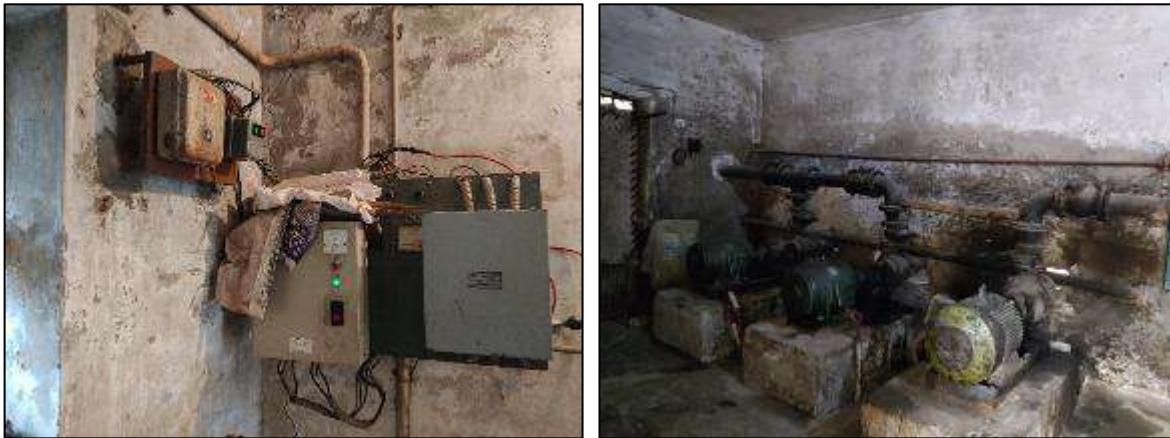
Figure 15: Electro-Mechanical components of Water Works Satellite Town
