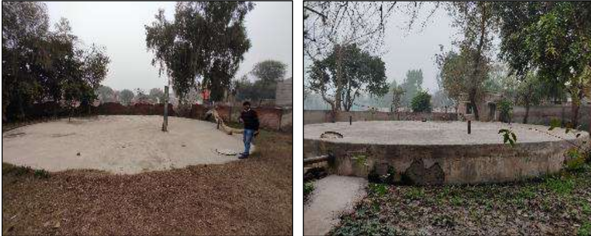
Figure 14: Ground Storage Tanks at Gill wala and Satellite Town Water Works
