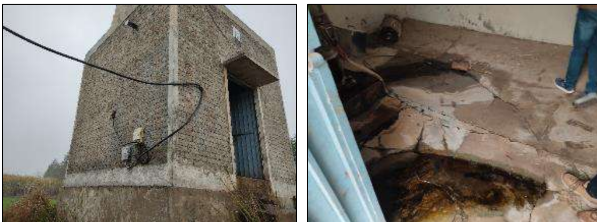
Figure 24: Bulged floor of a tube well in Kacha Shahpur
