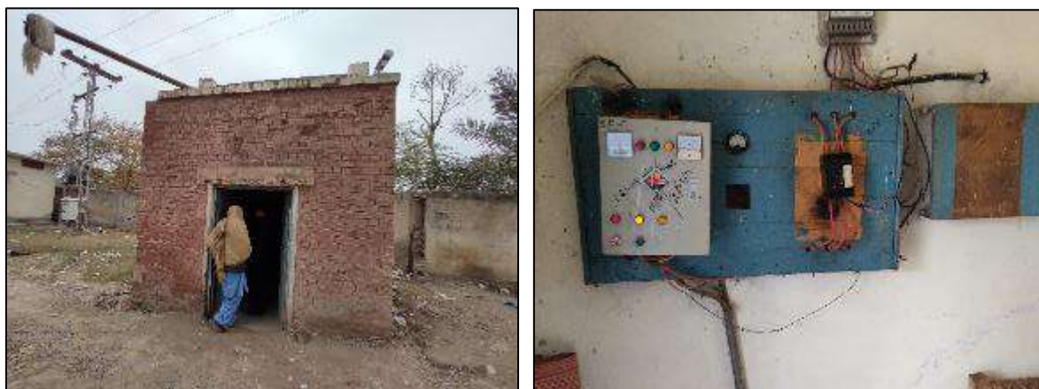
Figure 41: Civil structure and electrical components of tube wells in Mianwali City
