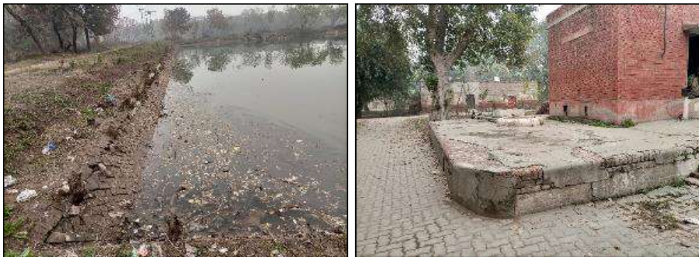
Figure 12: Damaged lining of pond and Damaged GST at Main Water Works Sargodha
