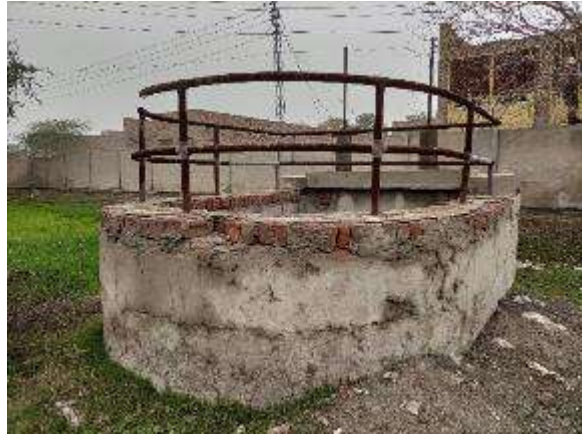
Figure 61: Outside Wet Well of Disposal Station
