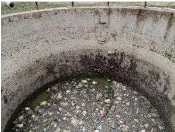
Figure 60: Inside Wet Well of Disposal Station Mandi Town
