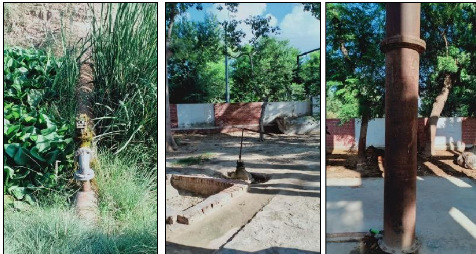
Figure 66: Condition of water distribution network in Bahawalnagar
