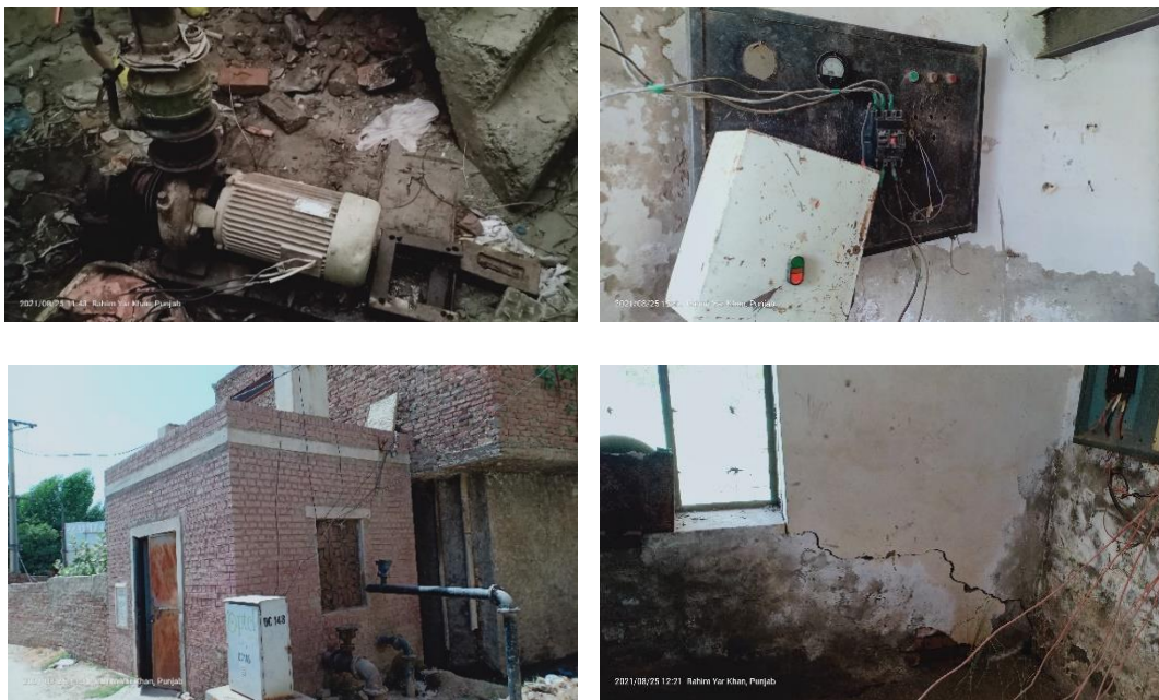
Figure 28: Glimpse of WSS Infrastructure Condition
