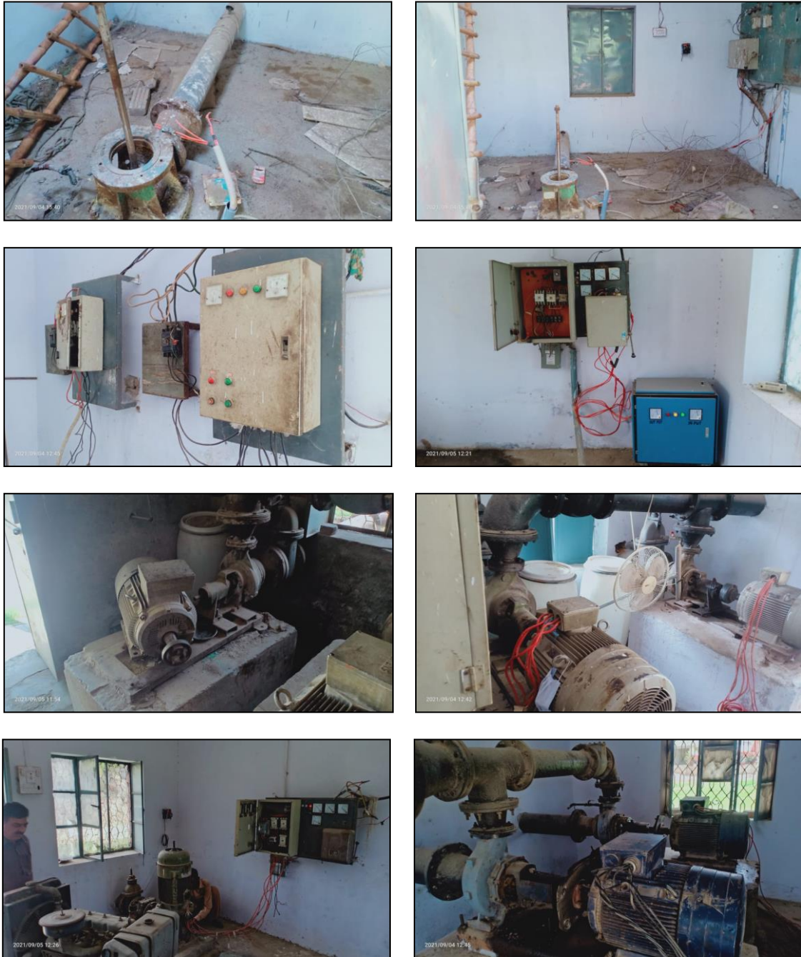
Figure 63: Condition assessment of water supply assets
