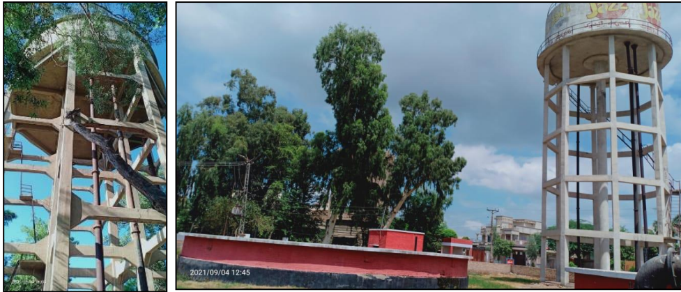
Figure 65: Overhead Reservoir and Ground Storage tank in Bahawalnagar
