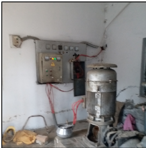
Water Works – Sialkot
