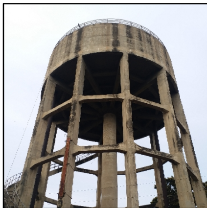
Water Works – Sialkot
