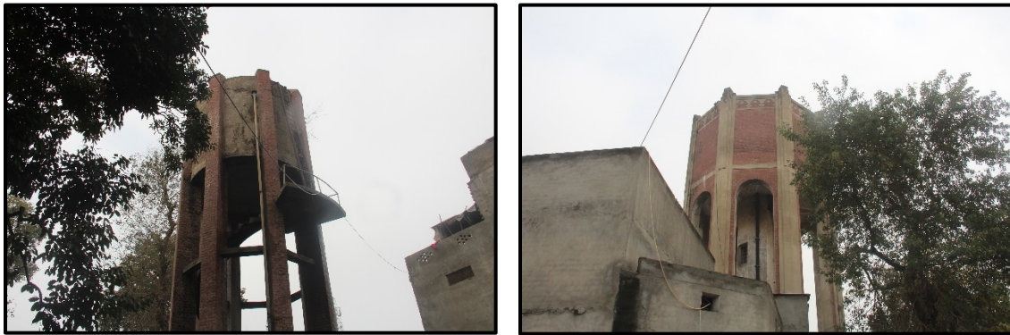
Figure 11: Existing OHRs in Narowal City (left: Old civil Hospital, Right: TMA Narowal)
