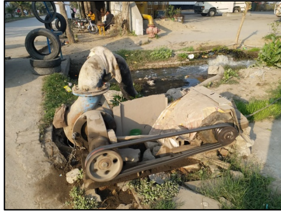
Pumping Station Gulshan Colony
