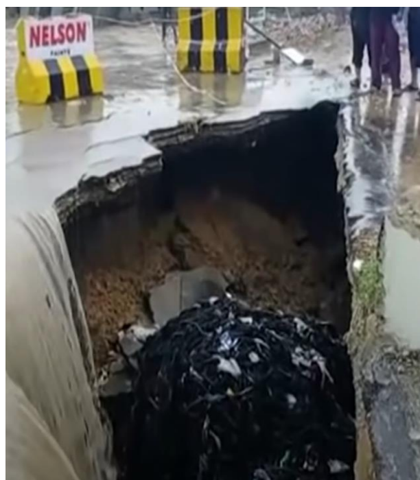
Figure 55. Damage to the Road Infrastructure in Karachi During 2020 Floods 90
